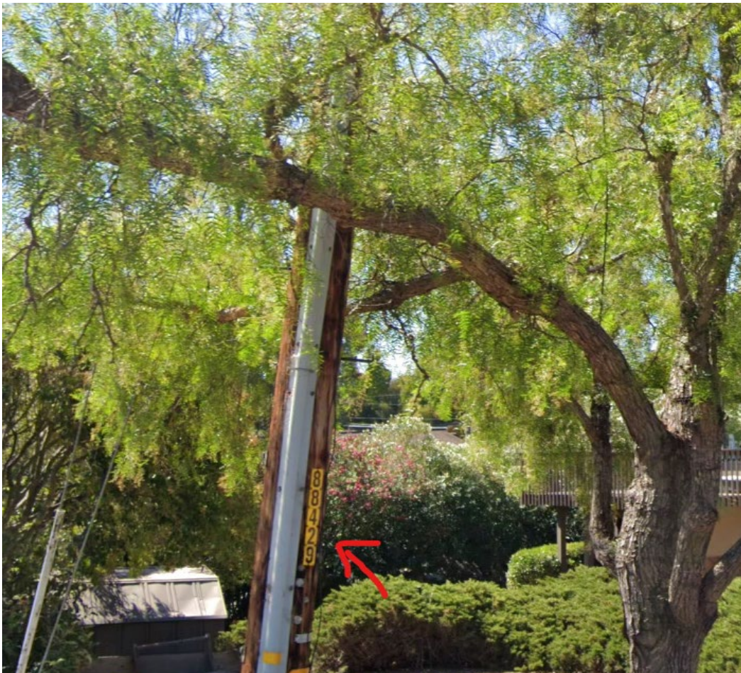
Image 1: Fuse ID 88429 / SAP Equipment # 100323195
