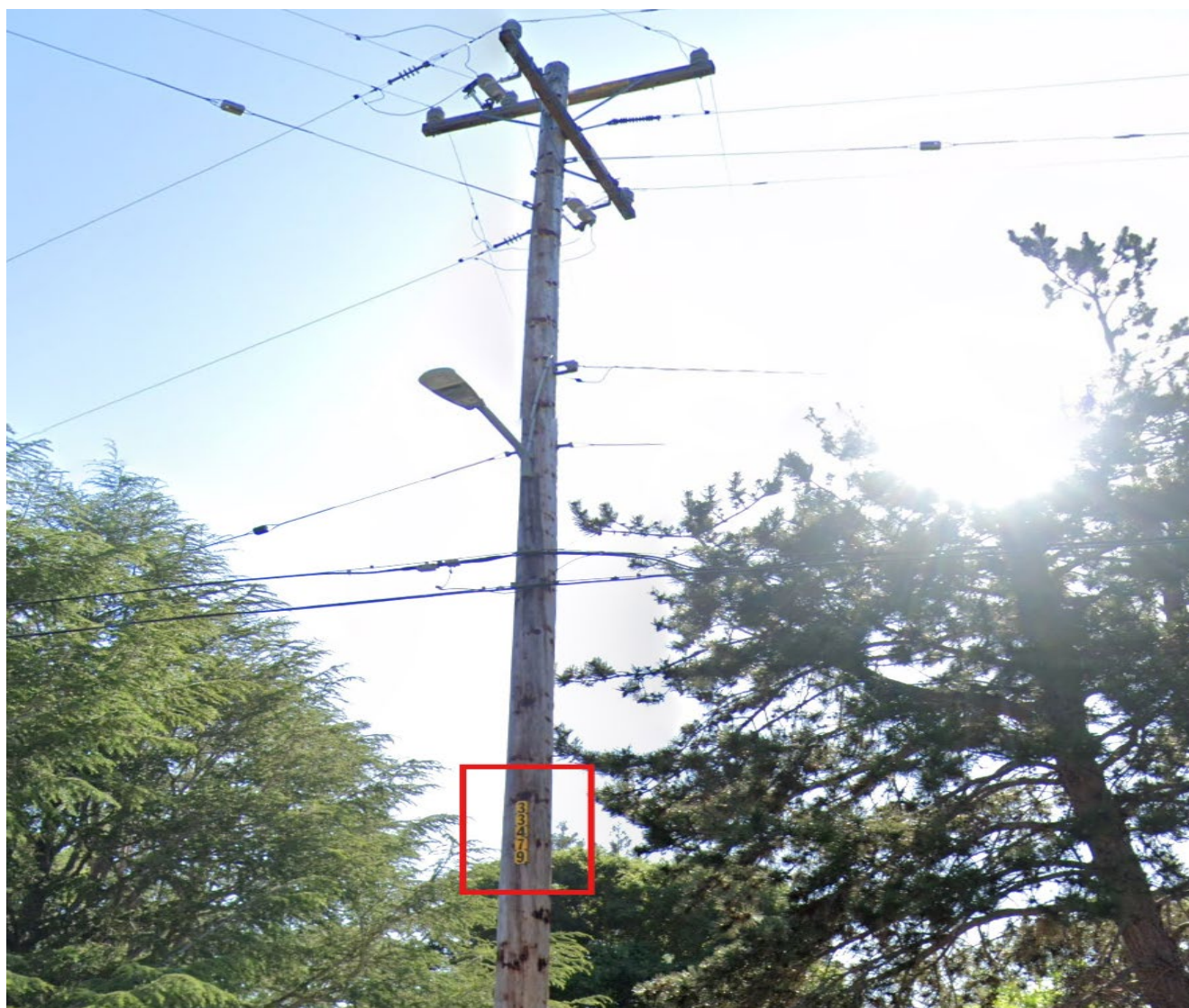
Image 1: Correct structure (pole ID 33479) with completed replacement Non-Exempt Expulsion Fuse with Solid Blades.
