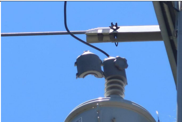
IA1img2: Open transformer bushing cover
