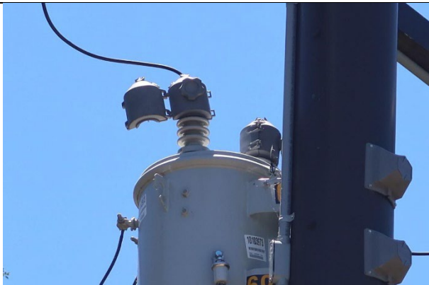
IA1img1: Open transformer bushing cover
