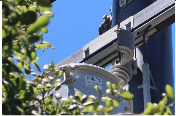
IA1Img4: Open transformer bushing cover
