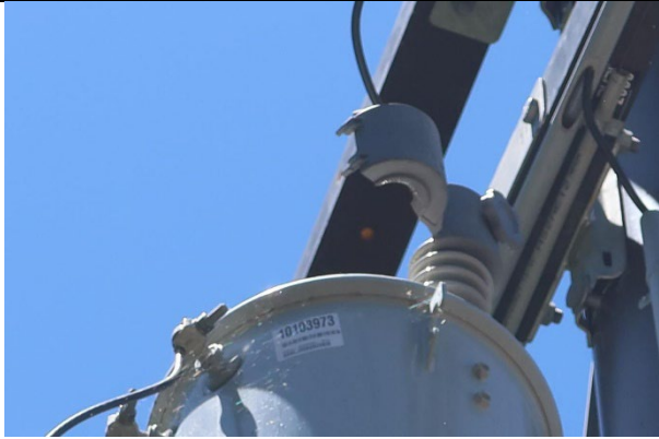
IA1Img3: Open transformer bushing cover
