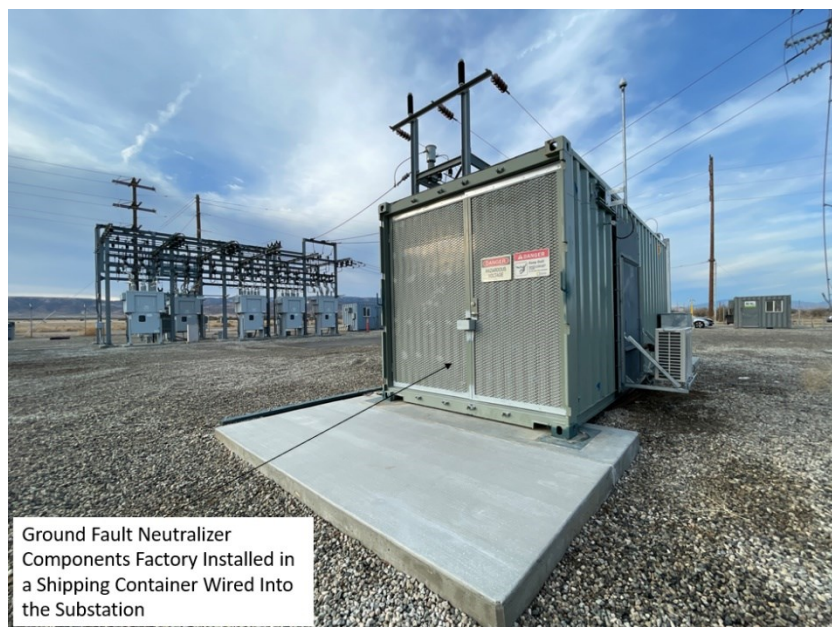
Figure SCE 8-07: Image of a Ground Fault Neutralizer
