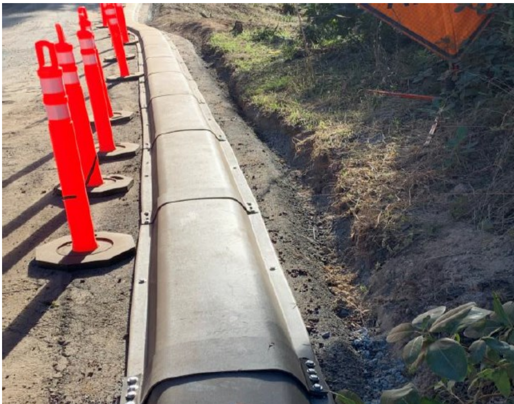
Figure SCE 8-04a: Cover Installed Over Cable Tray System from PG&E’s GLDS Pilot in Woodside
