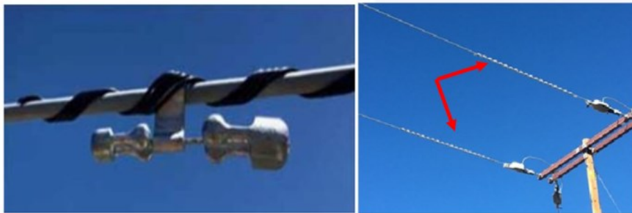
Figure SCE 8-02: Types of Vibration Dampers: Stockbridge Damper (left) and Spiral Damper (right)
