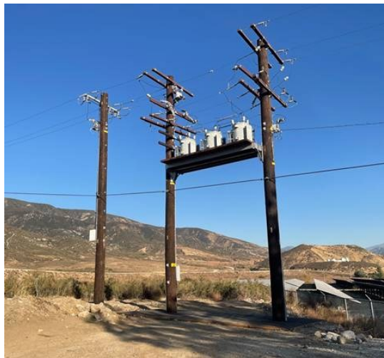
Figure SCE 8-08: Isolation (Iso) Bank Transformer (12kV to 12kV)
