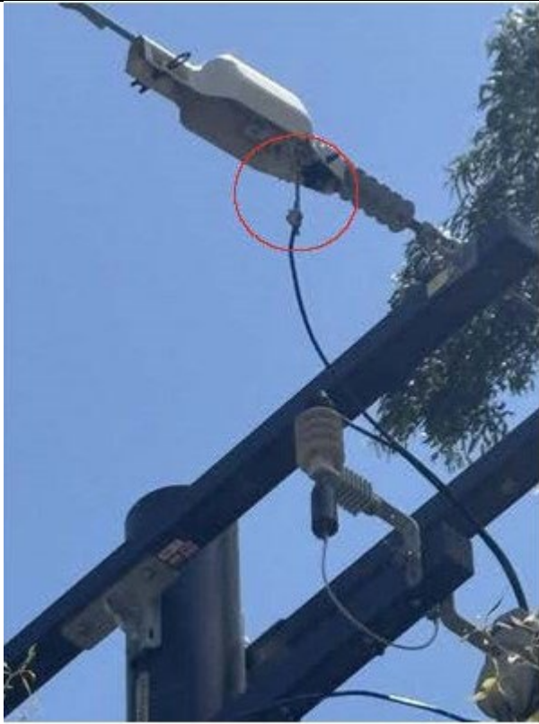
IA1Img1: Primary connection avian protection cover missing
