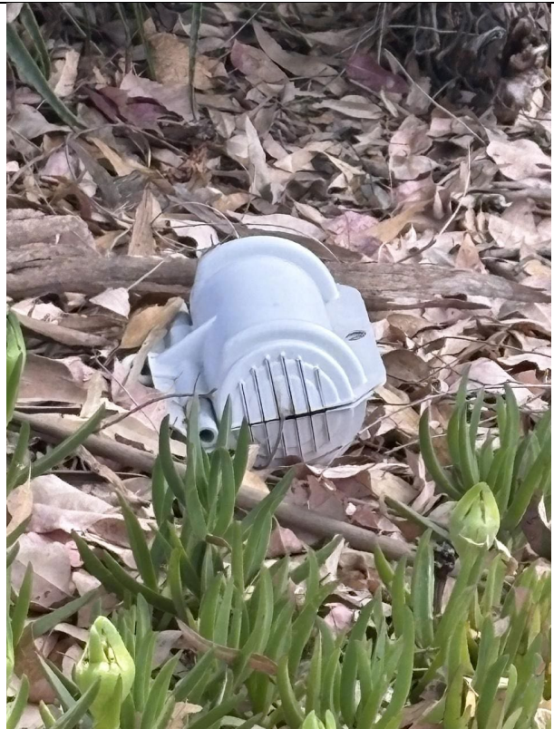
IA1Img4: Primary connection avian protection cover found on the ground
