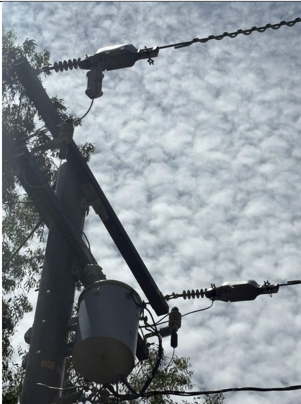
IA1Img3: Primary connection avian protection cover missing
