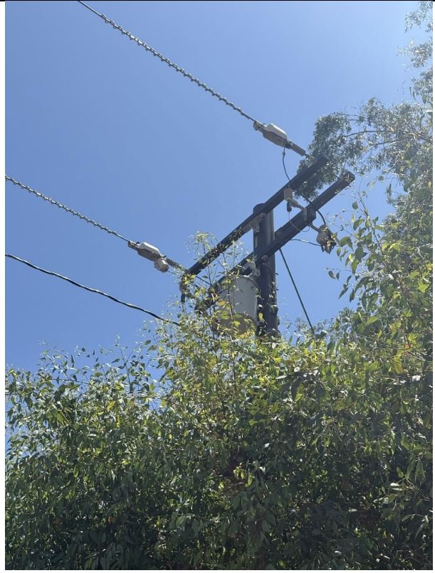
IA1Img2: Primary connection avian protection cover missing
