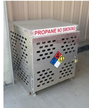
Compressed gas cylinder cage
