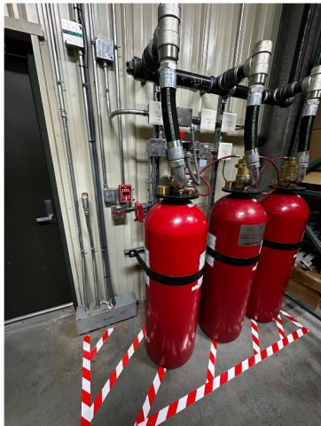
Spare Parts Building Suppression System
