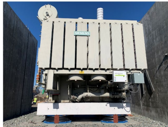
Pittsburg Substation- Transformer on Seismic Pad
