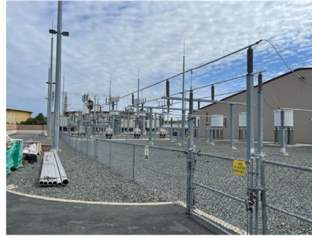
Pittsburg Station- Hardscaped AC Yard
