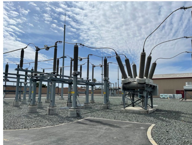
Pittsburg Station- Hardscaped HV Yard
