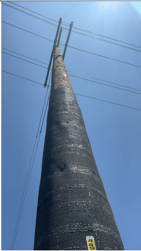
Item1IA1Img1: View showing no wildlife covers installed
