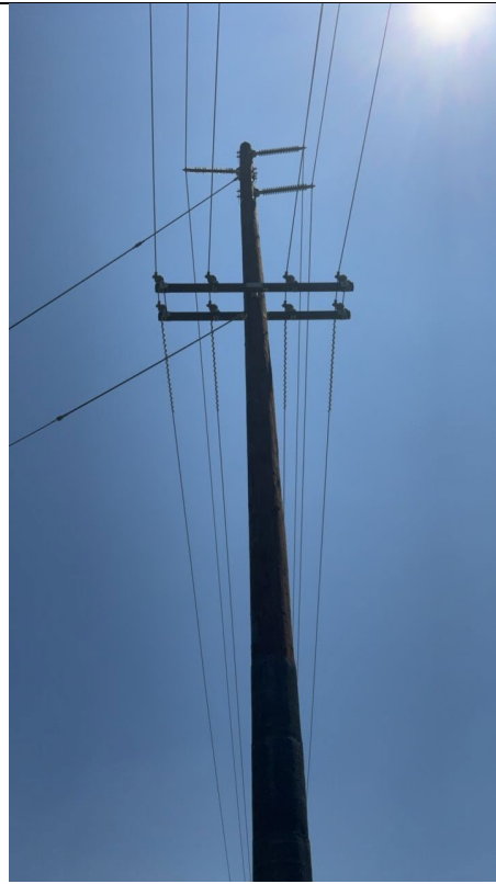
Item1IA1Img2: View showing no wildlife covers installed
