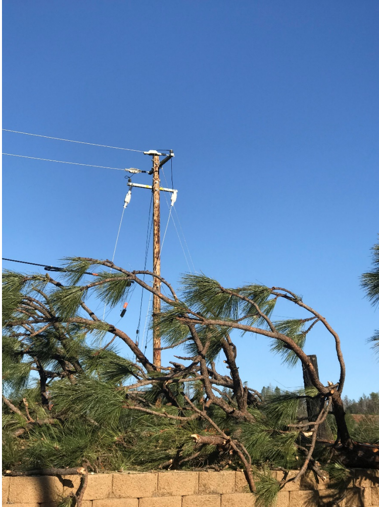
Figure 1: Failed tree and downed conductor.
