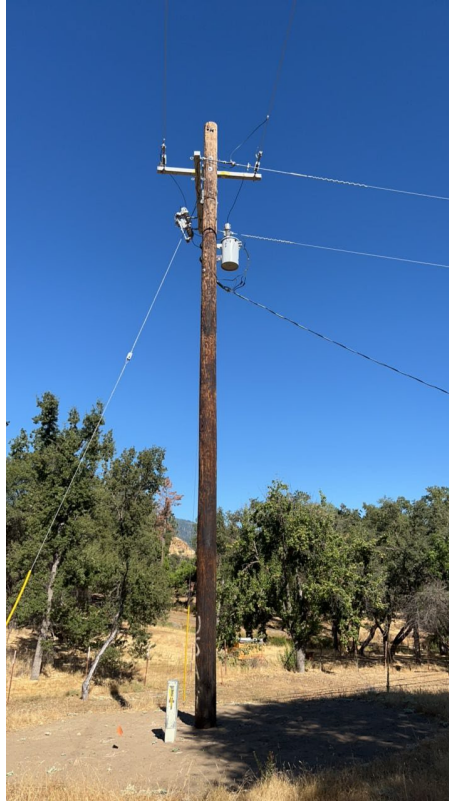
Item3GImg2: Overall pole east view
