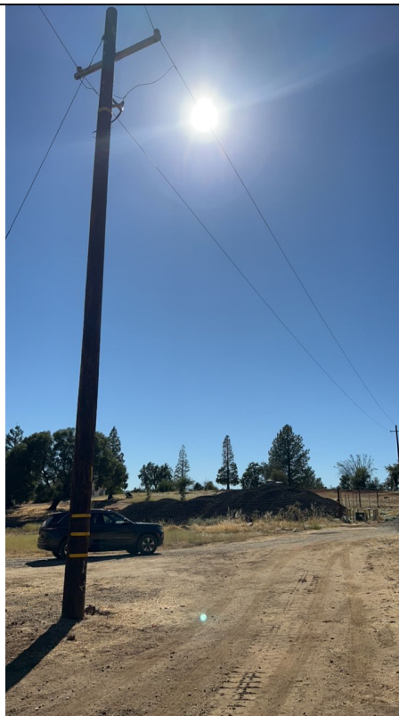
Item2GImg2: Overall pole with riser and underground pad mounted transformer in background
