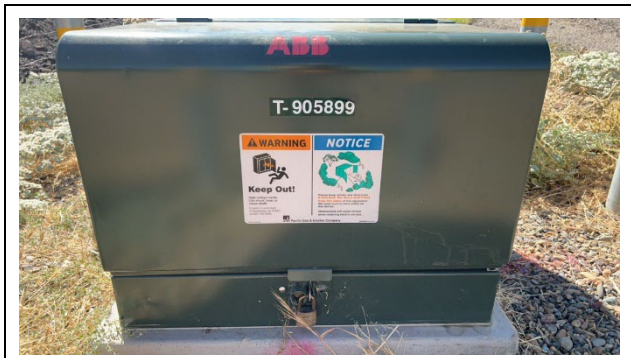
Item2IA1mg3: Nearest pad mounted transformer
