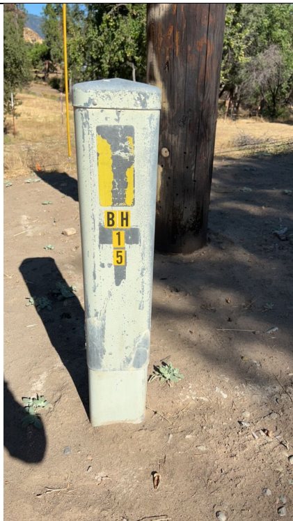
Item3GImg3: Equipment at base of pole
