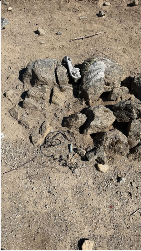
Item1GImg3: Abandoned dead end insulator
