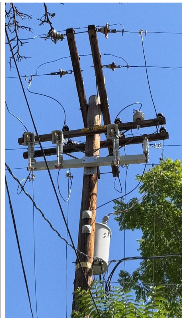
Item1IA1Img2: Three Exempt Non-Expulsion Branch Line Fuses and One Non-Exempt Expulsion Fuse to Transformer
