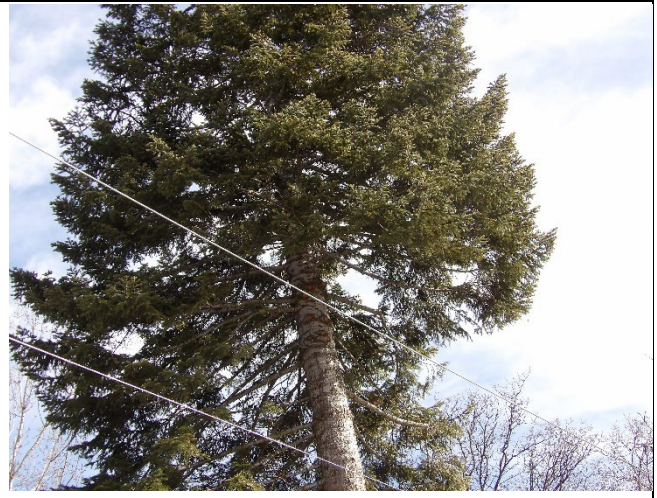
Item1Gimg6: South face view of white fir branches located within 12 feet of the distribution line. Photo taken December 19, 2024.
