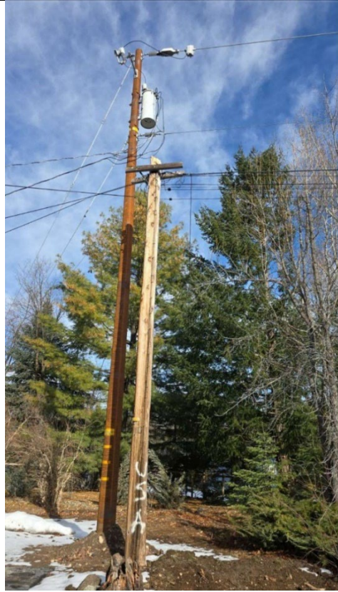
Item1GImg2: Overall Pole ID 084601 with equipment and surrounding vegetation. Photo taken December 19, 2024.
