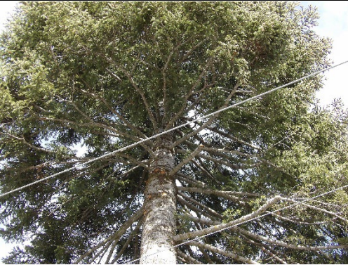
Item1GImg3: Close-up view of white fir branches located within 12 feet of the distribution line. Photo taken December 19, 2024.
