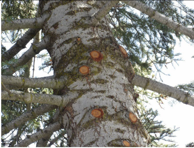
Item1Gimg5: Close-up view of the incomplete clearance work on the white fir. Photo taken December 19, 2024.
