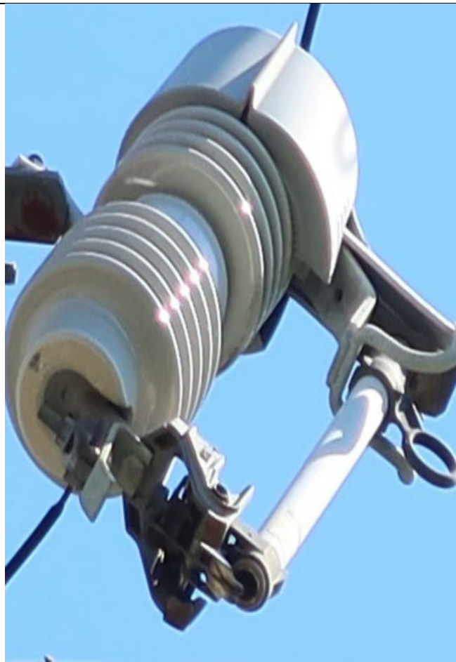
Item1IA1Img4: Close-up of non-exempt expulsion fuses.
