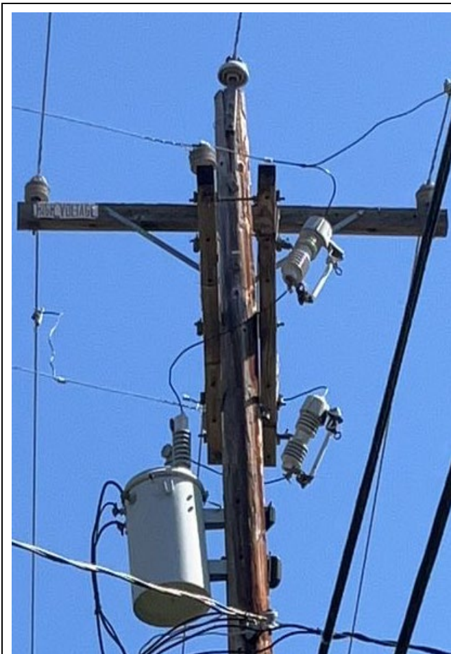
Item1IA1Img3: Non-exempt expulsion fuses.
