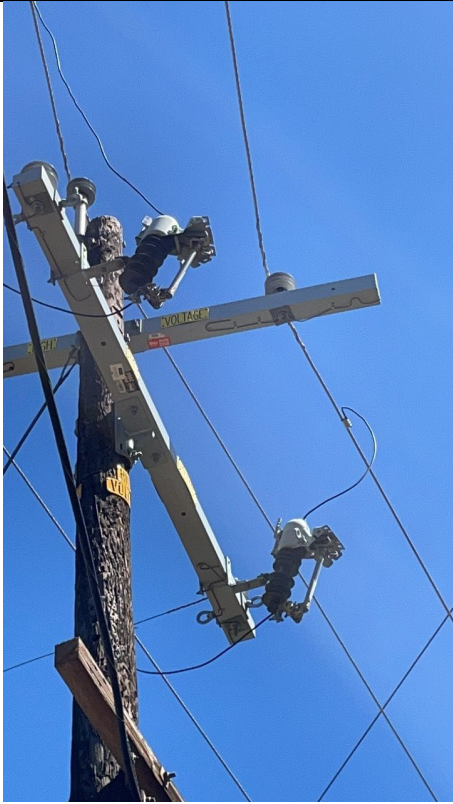
Item1IA1mg1: View of non-exempt expulsion fuses
