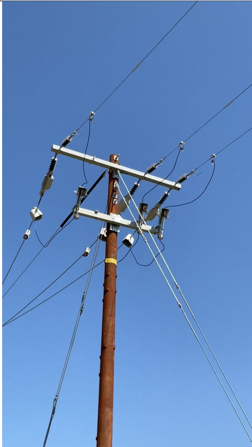
Item1IA1img3: Covered conductor was present to the north of the structure (Left), but no covered conductor was present to the south (Right)
