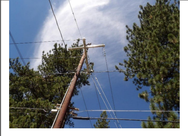
Item1IA1mg1: View of Adjacent Pole with No Primary Distribution Covered Conductor Continuing to Subject Pole
