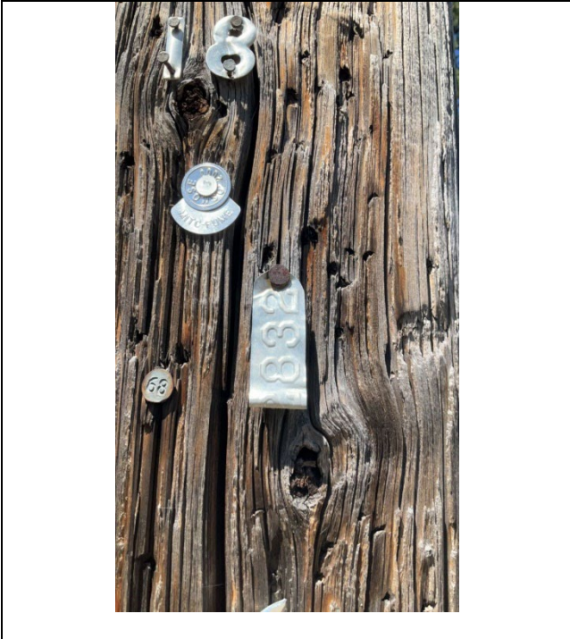
Item1G1mg1: Pole ID (Damaged)
