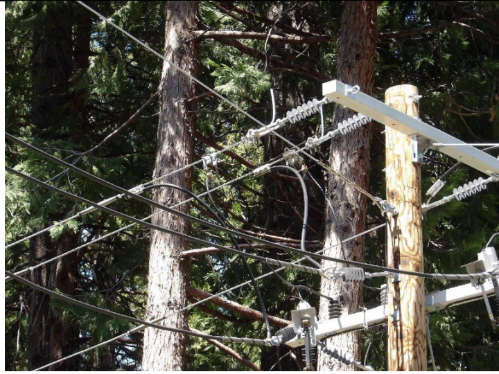
Item1IA1Img2: No Covered Conductor Present on Top Span
