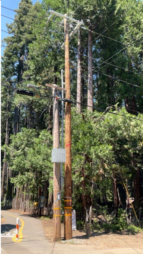
Item1Gimg2: Overall Pole, showing that covered conductor was not installed in a northerly direction from the pole as reported in the QDR.
