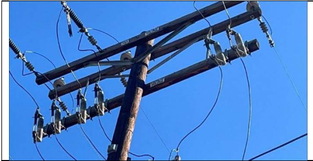
Item1IA1Img1: No avian protection covers
