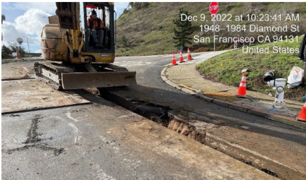
Photo 4: Scene of the excavation equipment and damage with cable protruding from the trench. Photo and timestamp of 10:23 a.m. by M Squared Construction. Black square added by investigator to redact M Squared Construction employee. (Exh. 20, pg. 24.)
