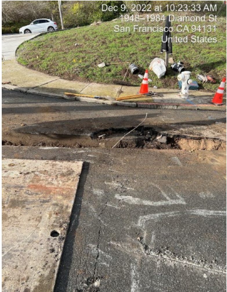
Photo 5: Trench with damaged cable protruding from trench looking west toward Diamond Heights Boulevard. Photo and timestamp of 10:23 a.m. provided by M Squared Construction. (Exh. 20, pg. 25.)
