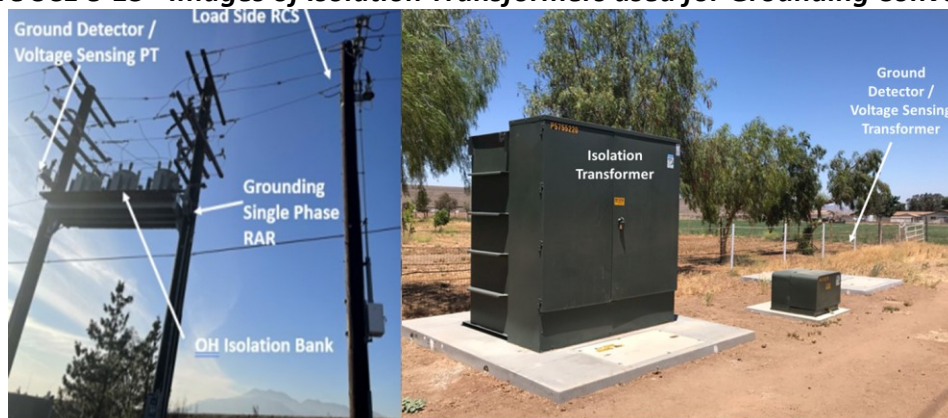
Figure SCE 8-13 - Images of Isolation Transformers used for Grounding Conversion
