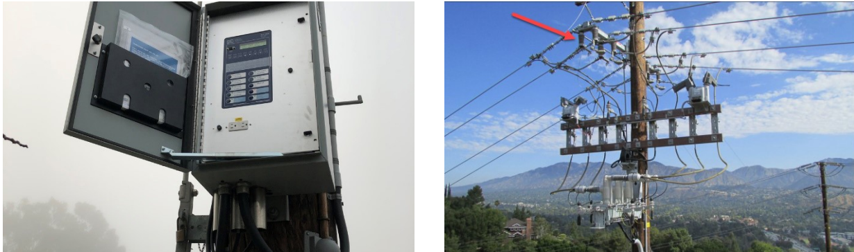
Figure SCE 8-15 - A Remote Control Box (left) and Remote Automatic Recloser (RAR) Switch (right)
