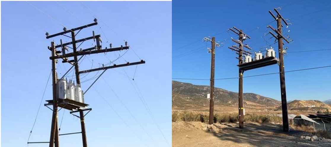
Figure SCE 8-12 - Pole Top Step Down (33kV to 12kV) Transformer (left) and Isolation (Iso) Bank Transformer (12kV to 12kV) (right)
