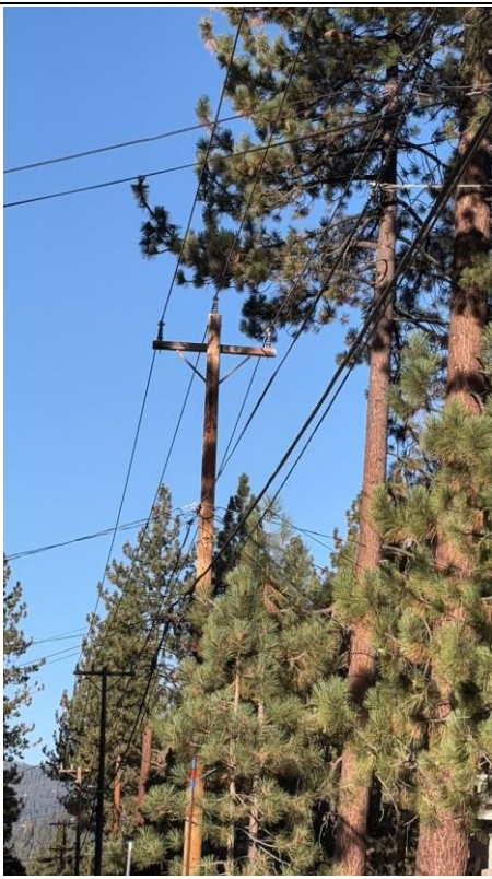
Item1IA1mg1: View of Jeffrey pine with limb that could contact both conductors and cause arcing between the two phases. Evidence of previous vegetation work, including limb removal on the subject tree. Photograph taken from Cutthroat Avenue facing west. Tree is north of pole 286848. Zoomed.
