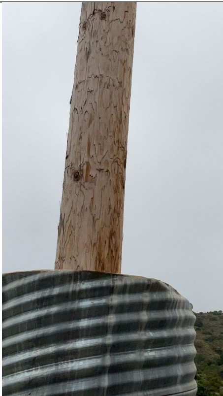
Item2GImg1: Missing Pole ID
