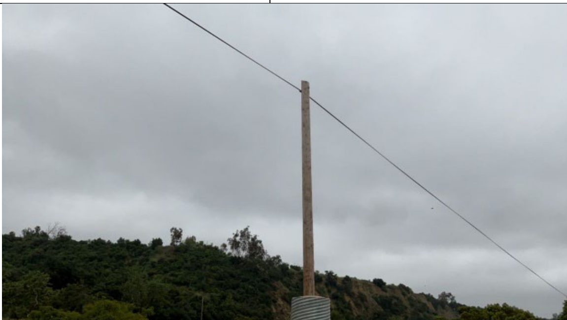
Item2IA1Img1: No covered conductor present
