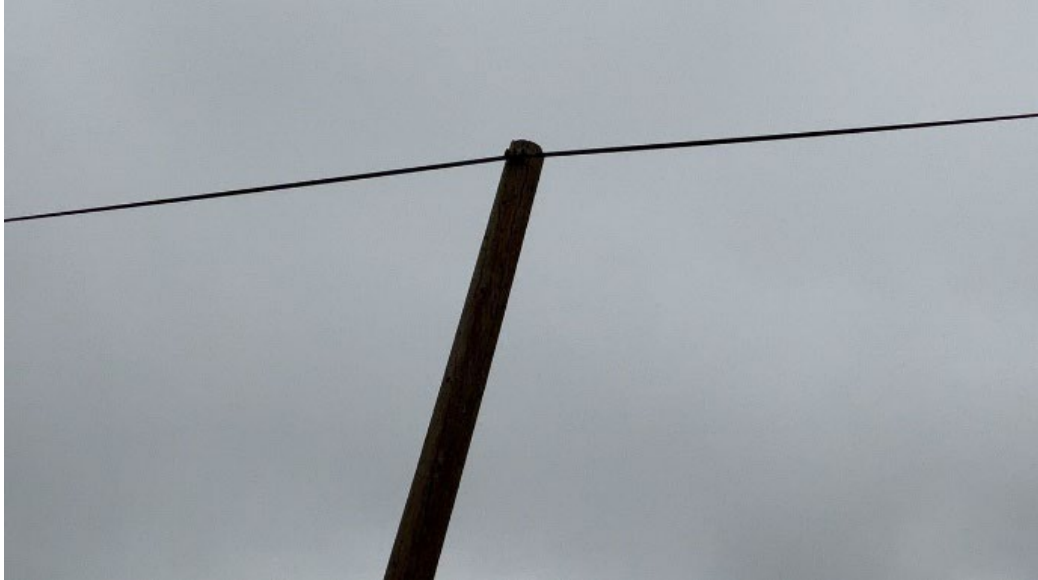
Item1IA1mg1: No covered conductor present
