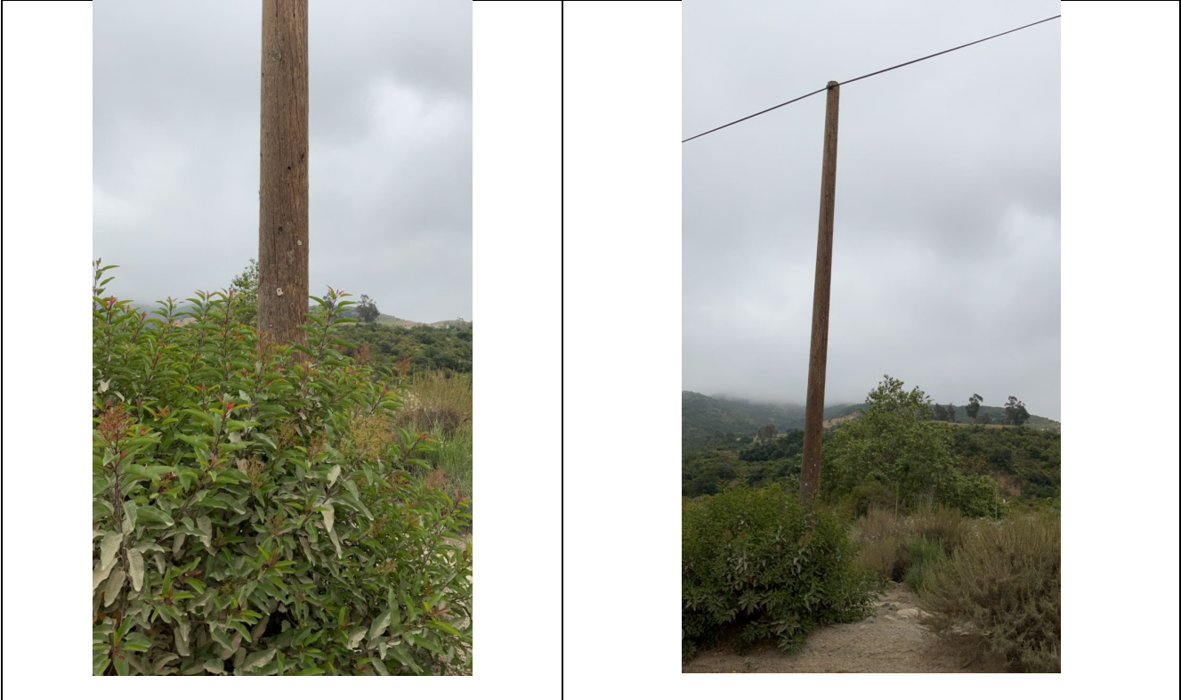
Item1G1mg1: Missing Pole ID
