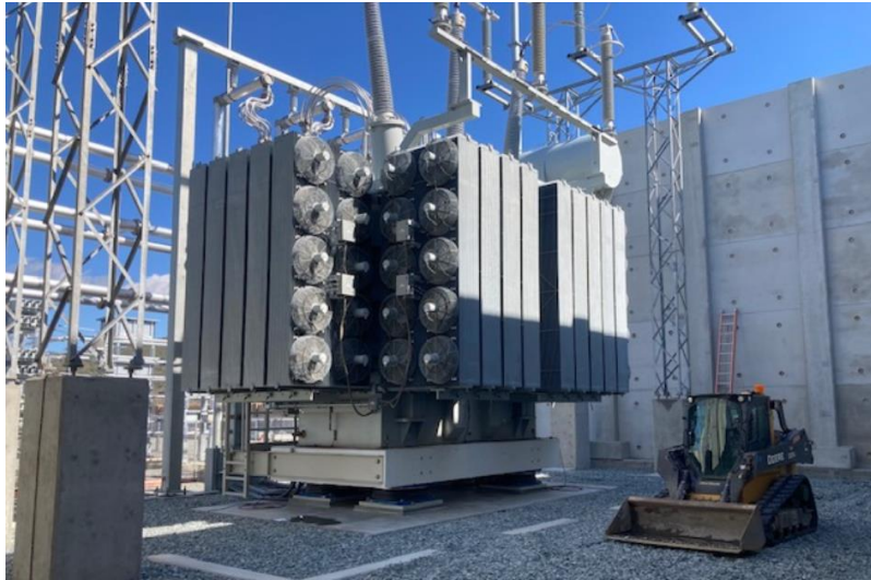
Figure HWT 8.1.2-3. Transformer Seismic Isolation Pad
