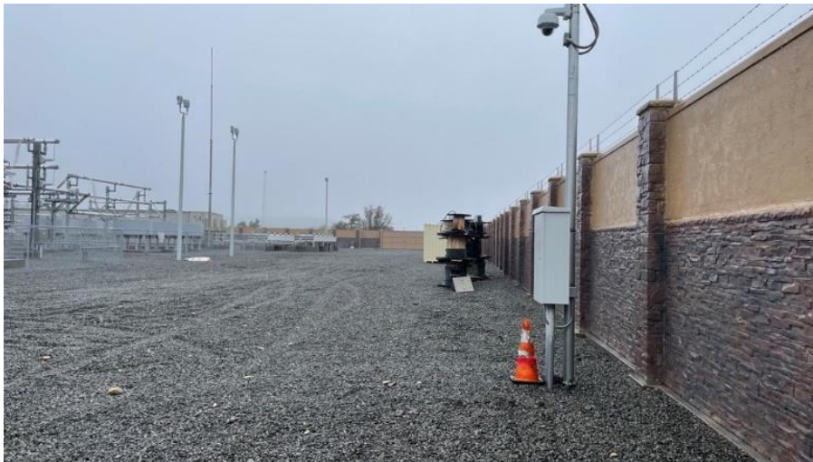
Figure HWT 8.3.2-1. Example of Site Camera
