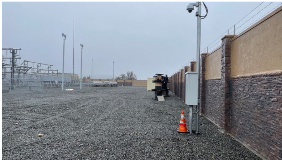
Figure HWT 8.3.2--1. Example of Site Camera
