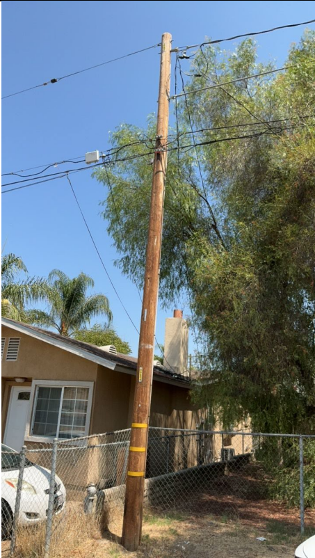
Item1Gimg1: Overall pole.
