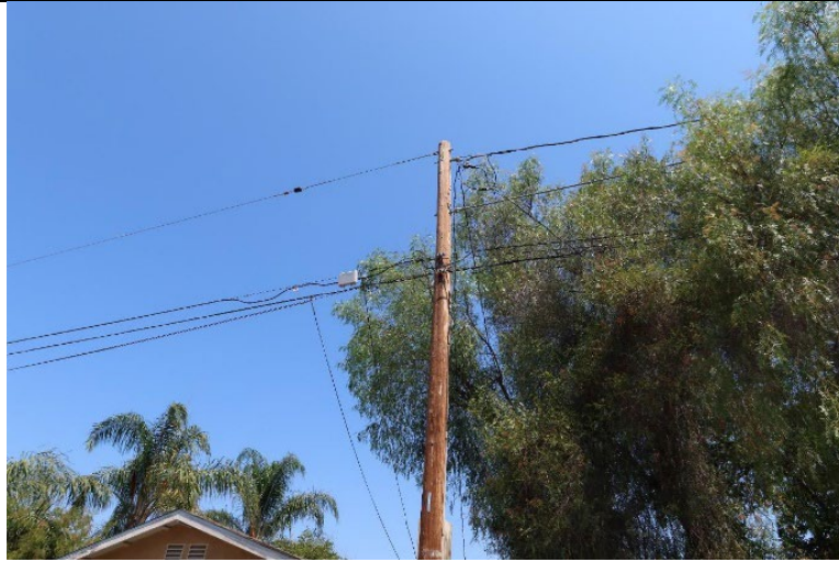
Item1IA1Img1: View of secondary distribution pole where covered conductor installation was reported as installed.
