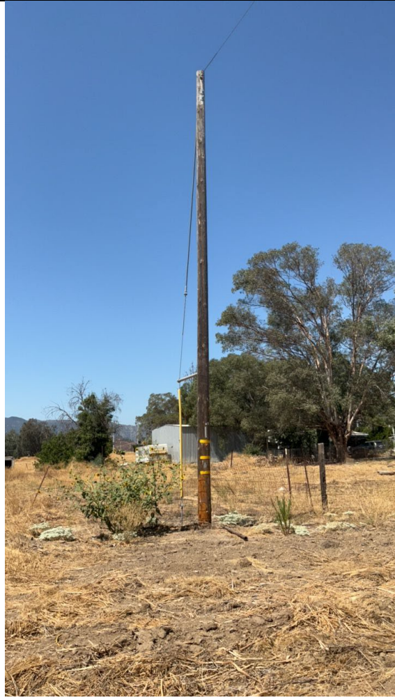
Item1IA1Img1: No covered conductor installed.
