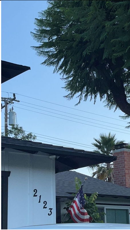
Item1IA1mg3: California palms breaking minimum clearance requirements. Photograph was taken from the north side of the sidewalk along Cheam Avenue facing 355.8 degrees north.
