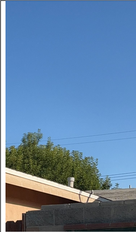
Item1IA1mg1: Ash tree breaking minimum clearance requirements. Photograph was taken facing 328.9 degrees northwest from Ish Drive.
