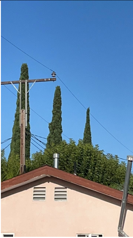
Item1IA1img3: Ash tree breaking minimum clearance requirements. Photograph was taken facing 241 degrees west from Buyers Street. Conductors are the same height as each other in this photograph.
