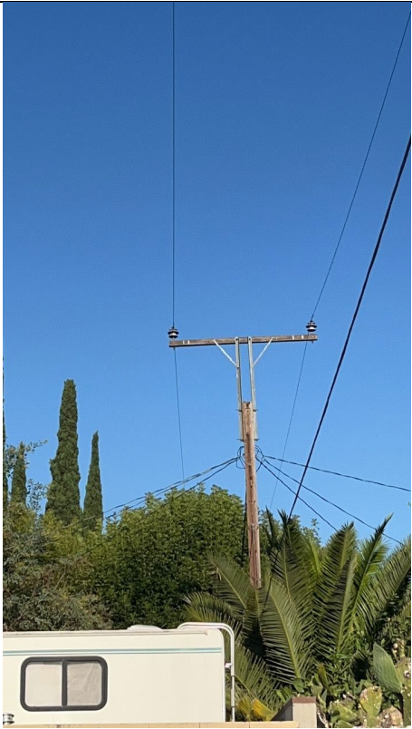
Item1IA1mg2: Ash tree breaking minimum clearance requirements. Tree appears to be growing directly under the lines and has evidence of previous vegetation management work. Photograph was taken facing 263 degrees west from Buyers Street.
