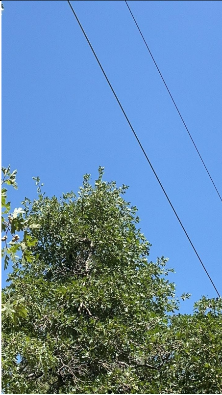
Item1IA1img2: Zoomed in image of oak tree branches of concern within 72 inches of the conductor. Inspector took the image 341.3 degrees north of the conductor.
