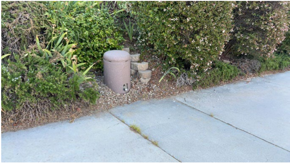
Item1IA1img1: Closeup of irrigation device
