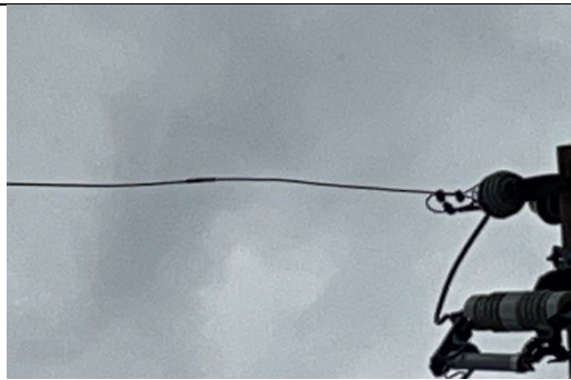
Item1IA1mg2: Close up of existing bare conductor.
