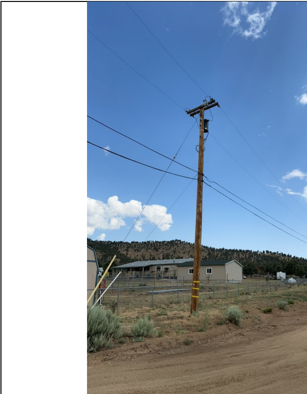
Item1G1mg1: Overall pole.
