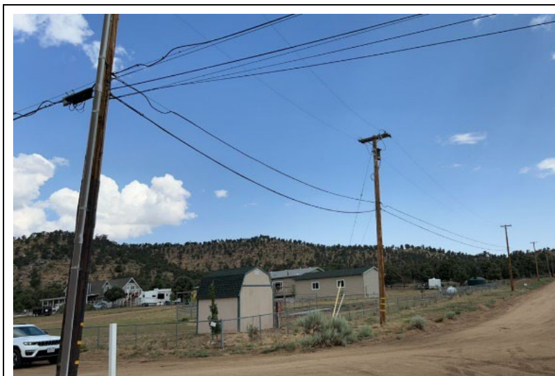
Item1IA1img3: Overall photo showing five spans where covered conductor was reported as installed.
