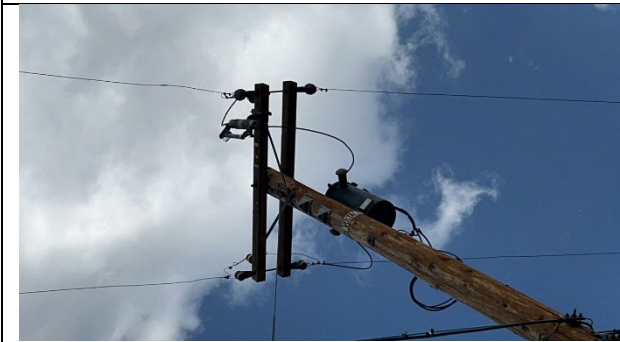
Item1IA1mg1: Overall primary level showing no cover conductor installed.
