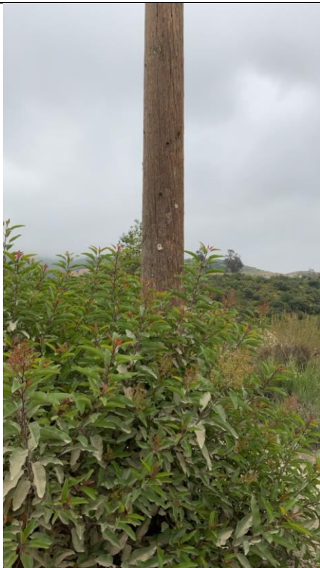
Item2GImg1: Missing Pole ID
