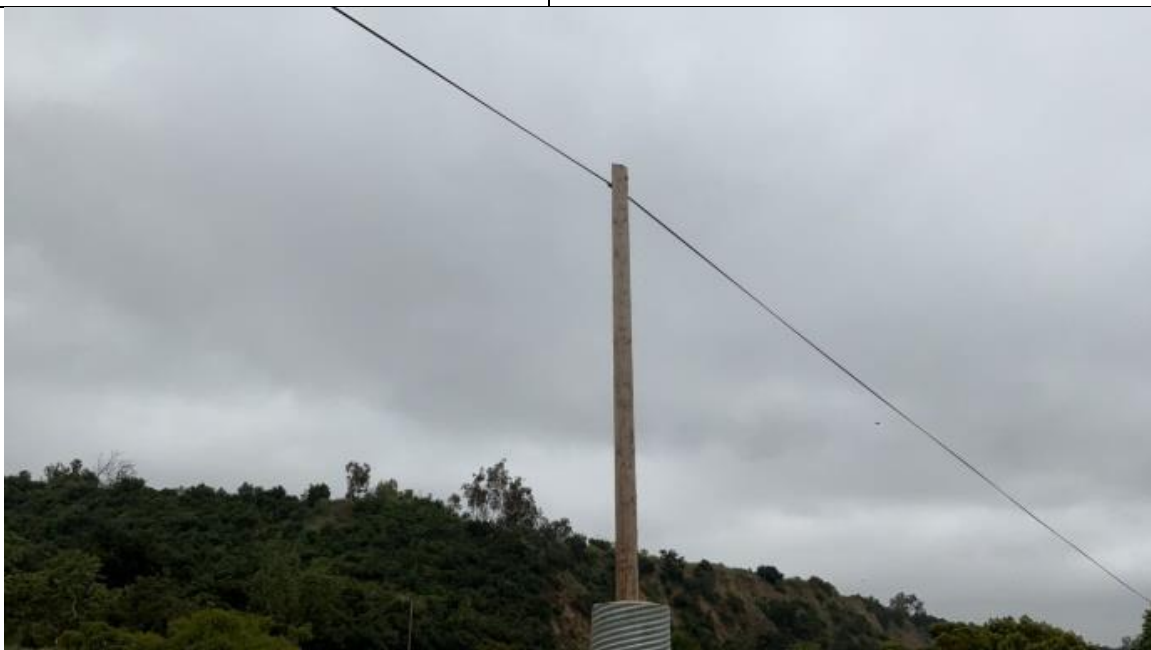
Item3IA1Img1: No covered conductor present
