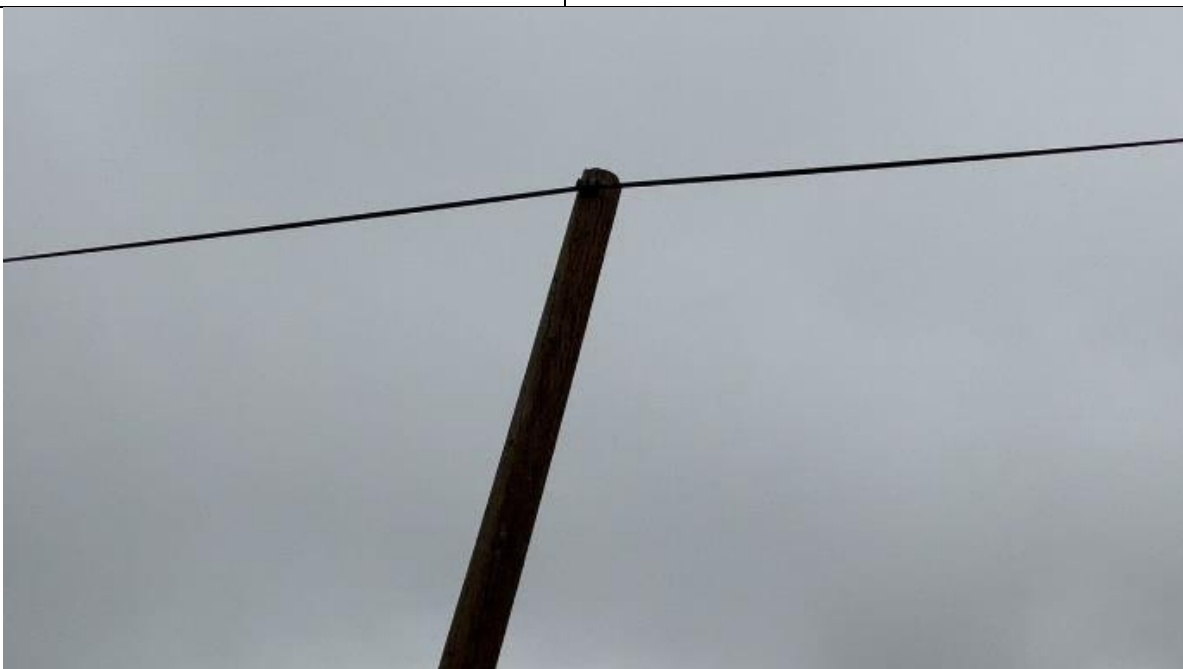
Item2IA1Img1: No covered conductor present
