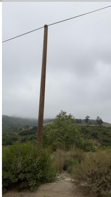
Item2GImg2: Overall Pole
