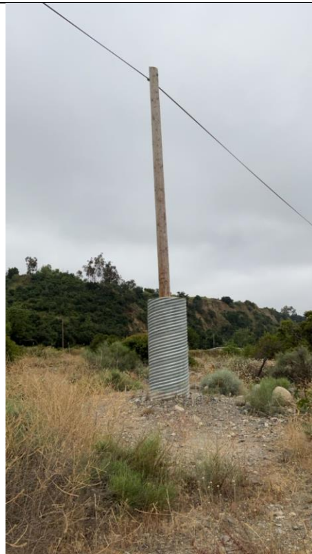
Item3GImg2: Overall Pole
