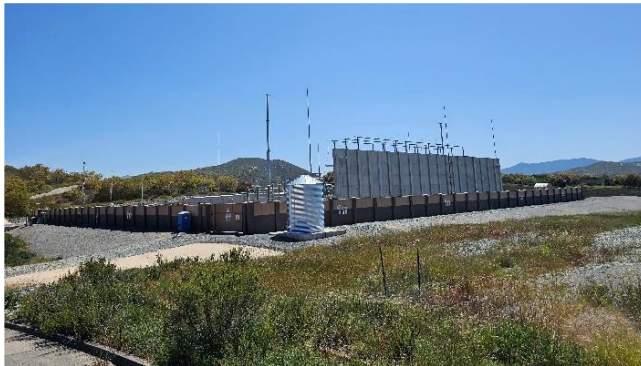
View of Substation facing East showing firebreak & water tank
