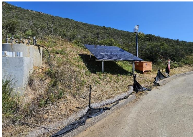
Solar Panel, Camera, and Control box
