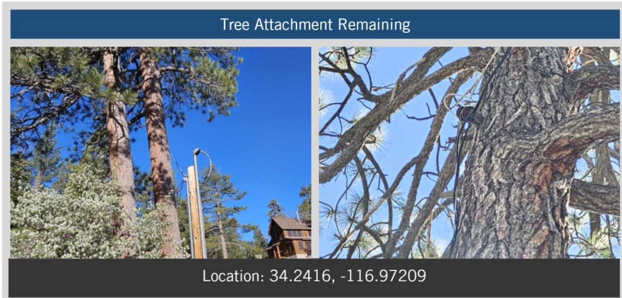
Figure 8: Secondary Conductor Tree Attachment Remaining
