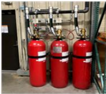
Figure 10 – Extinguishing Agent Cylinders
