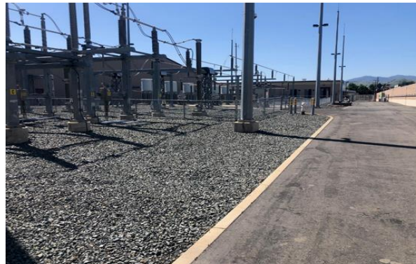
Figure 28 - Fire Lane and 180 kV Yard
