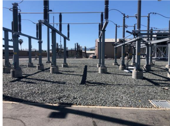
Figure 30 - 230 kV Risers & Circuit Breakers
