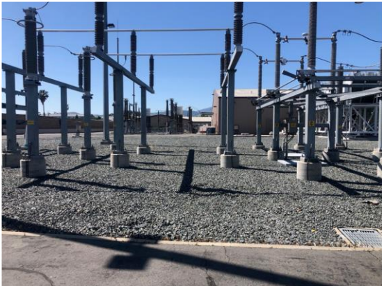
Figure 31 - Risers and Circuit Breakers with Transformers in Background
