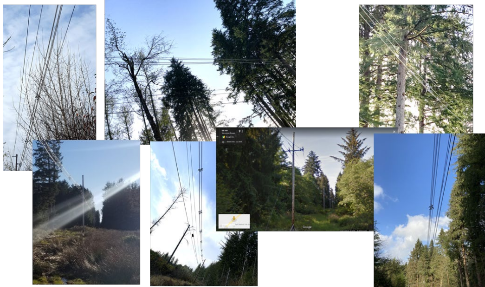
Figure F-5 PacifiCorp Covered Conductor Effectiveness Examples
