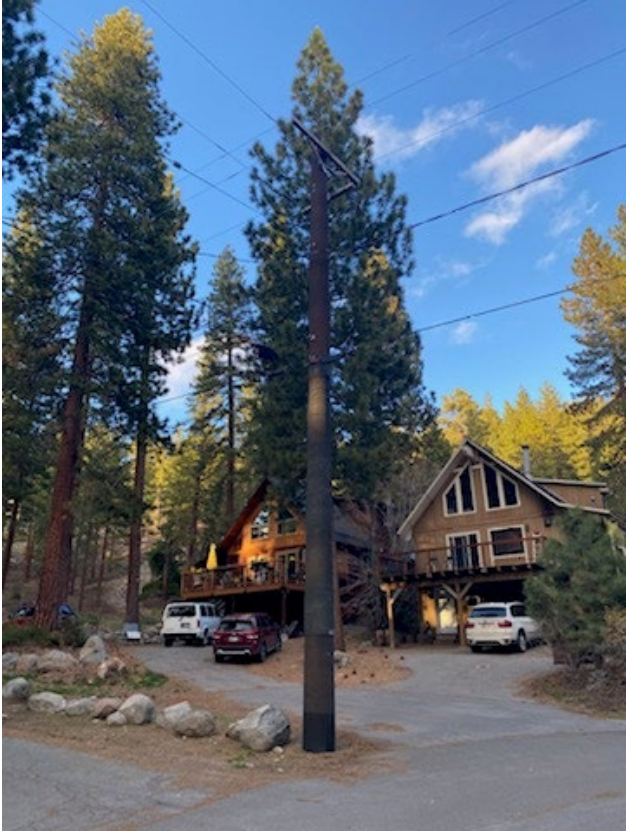
Photo showing pole #291897:
