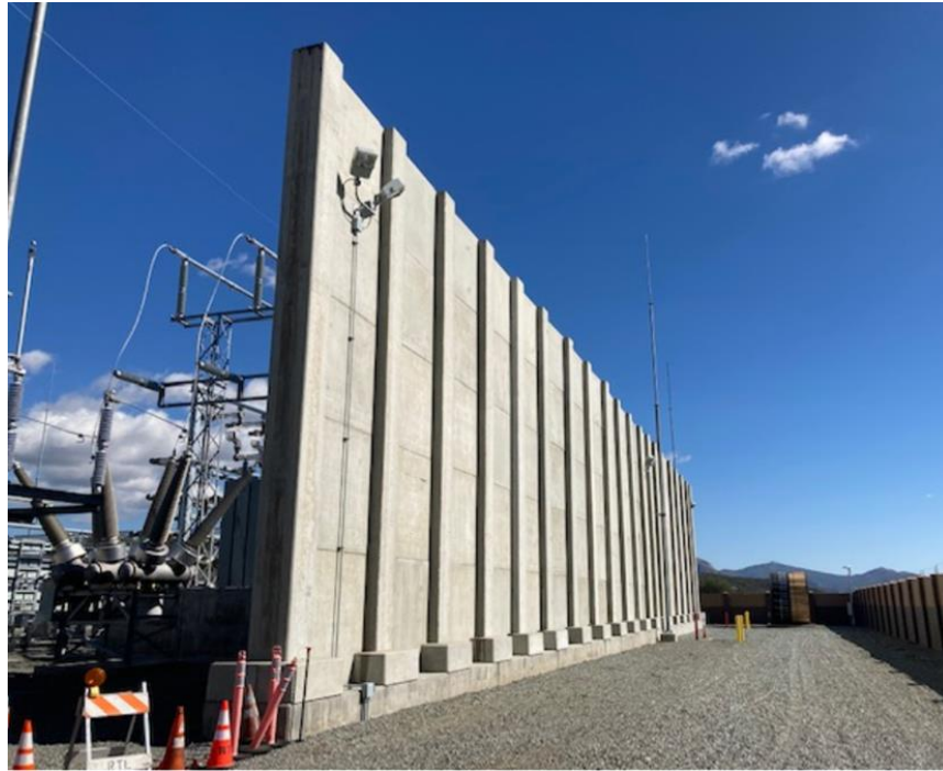
Figure HWT 8.1.2- 1. Transformer Fire Barrier Wall
