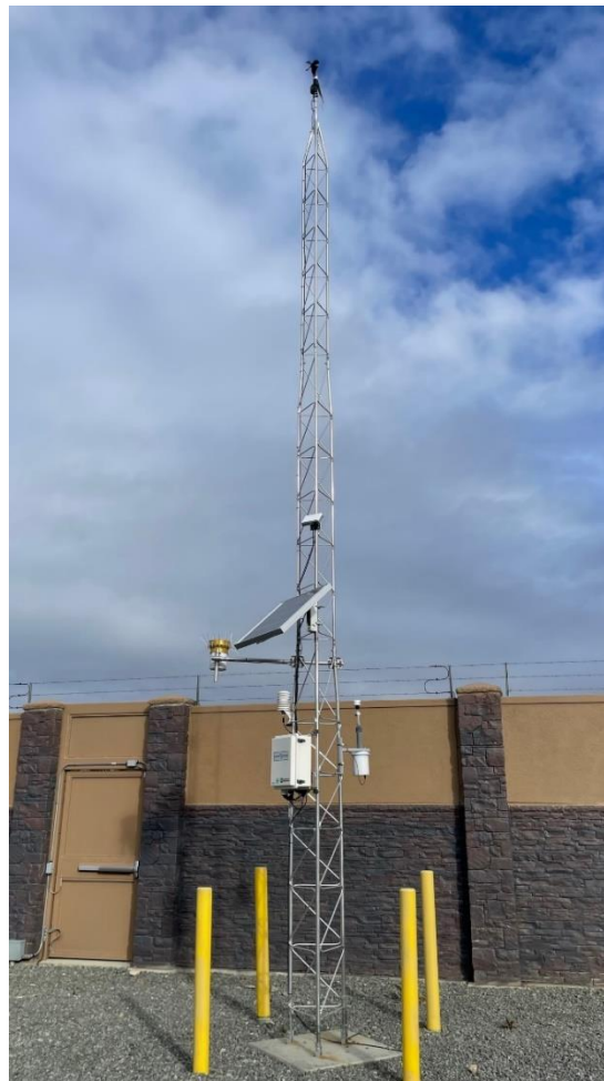
Figure HWT 8.3.2- 2. Weather Station
