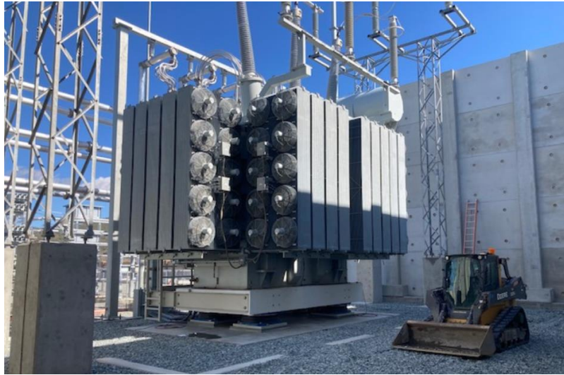
Figure HWT 8.1.2- 3. Transformer Seismic Isolation Pad
