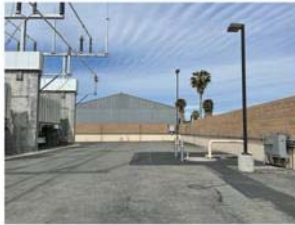
Figure TBC 8.1.2- 3. Hardscaped AC yard
