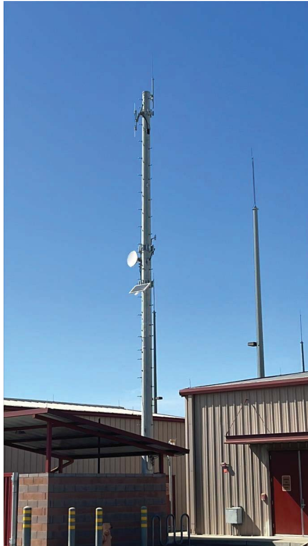
Figure TBC 8.3.2- 1. Weather Station at the Pittsburg Converter Station
