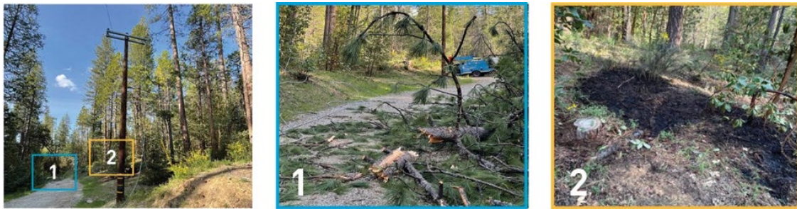
Figure F-3 PG&E Covered Conductor Effectiveness – Example 2
