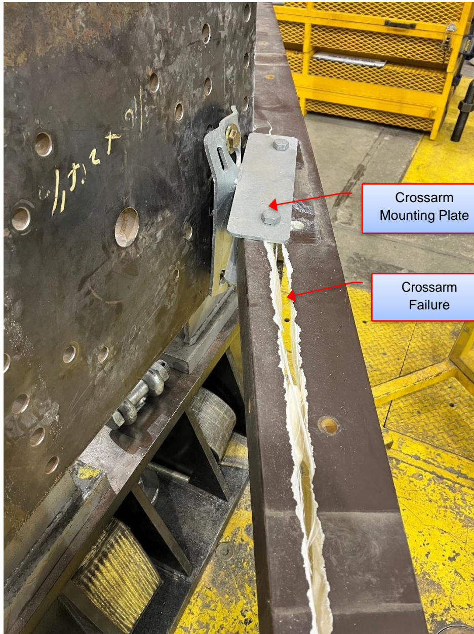
Figure 6-27: Sample 7.3 – Failure Location
