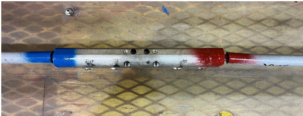
Figure 3-5: [REDACTED] Installed on 15 kV 1/0 AWG, 6/1 ACSR
