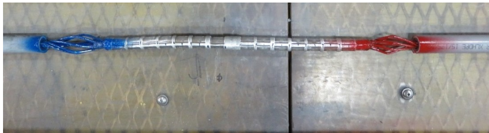
Figure 3-3: ██████ installed on 35 kV 1/0 AWG, 6/1 ACSR
