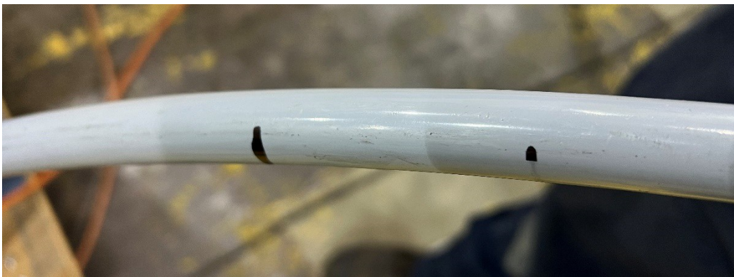
Figure 6-34: Sample 3K.1.3 - 17 kV, 1/0 AWG ACSR Condition after Test
