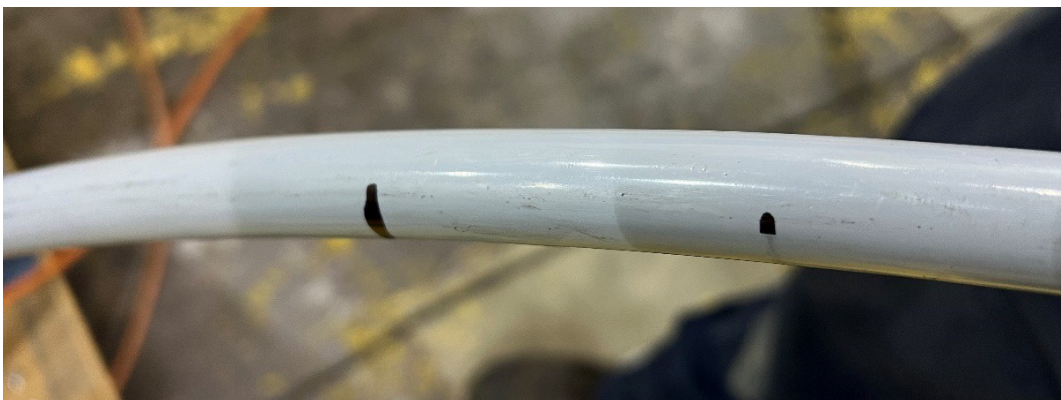
Figure 6-30: Sample 3K.1.3 - 17 kV, 1/0 AWG ACSR Condition after Test
