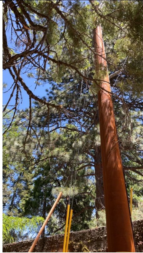
Item1IA1Img2: Dead branches are within the 10-foot radius of the pole and approximately 10 feet from the ground.
