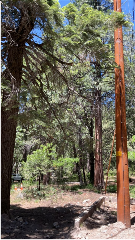
Item1IA1Img1: Dead branches are within the 10-foot radius of the pole and approximately 10 feet from the ground.
