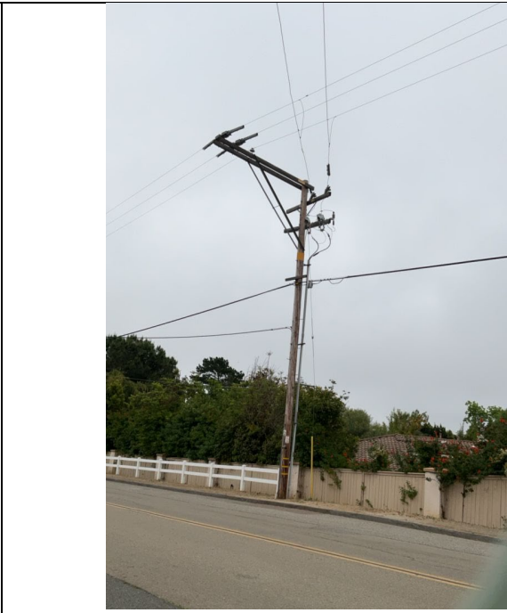
Item1GImg2: Overall Pole
