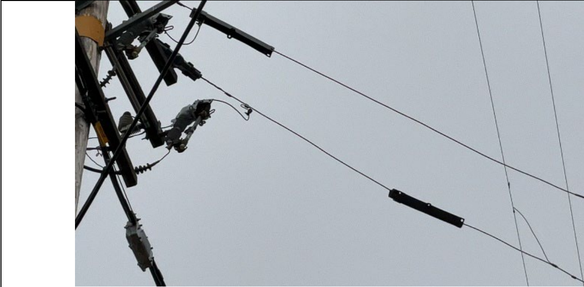
Item1IA1Img1: Dislodged avian protection cover
