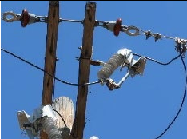
Item7IA1Img2: View of expulsion fuse
