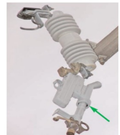
S&C Fault Tamer Fuse - Open
