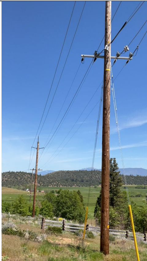
Item3IA2Img1: View to the north showing covered conductor ending at subject pole and bare conductor extending northward.
