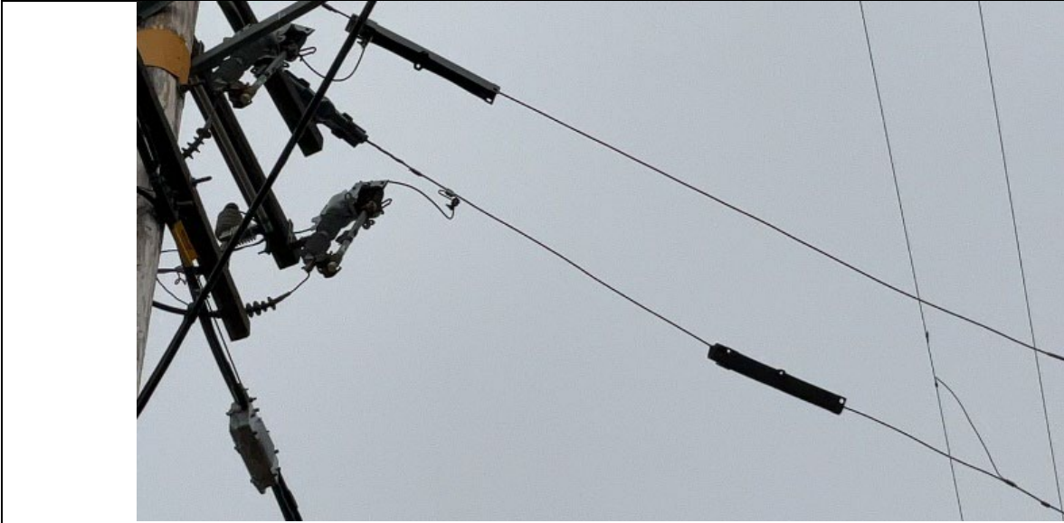
Item1IA1Img1: Dislodged avian protection cover
