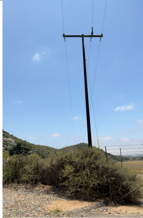
Item5GImg2: Overall pole
