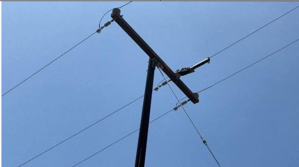
Item5IA1Img1: Missing avian protection cover on one side
