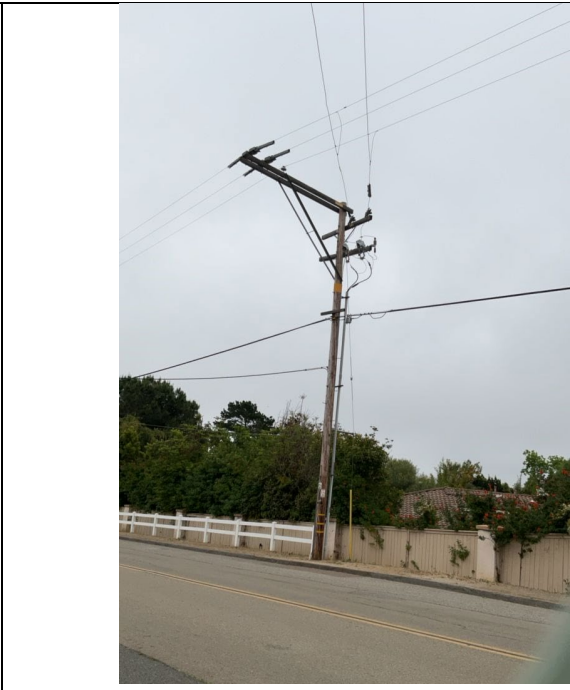
Item1GImg2: Overall Pole
