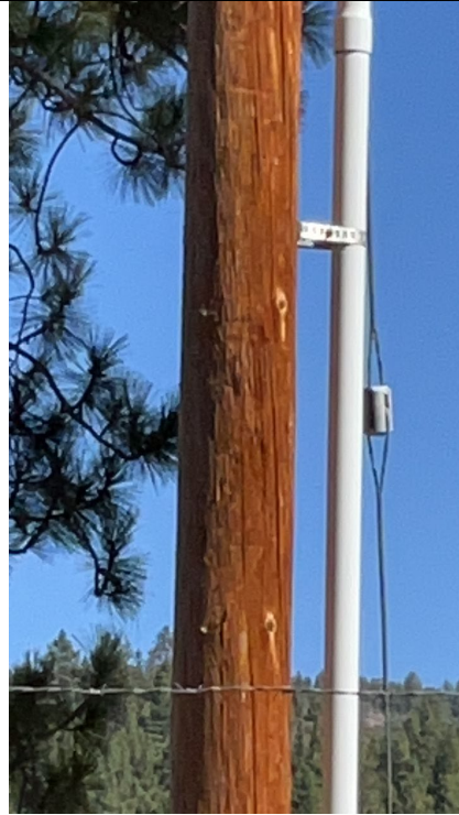
Item2GImg2: Pole ID not on the pole.
