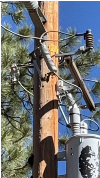
Item2GImg3: Close-up view of expulsion fuses.
