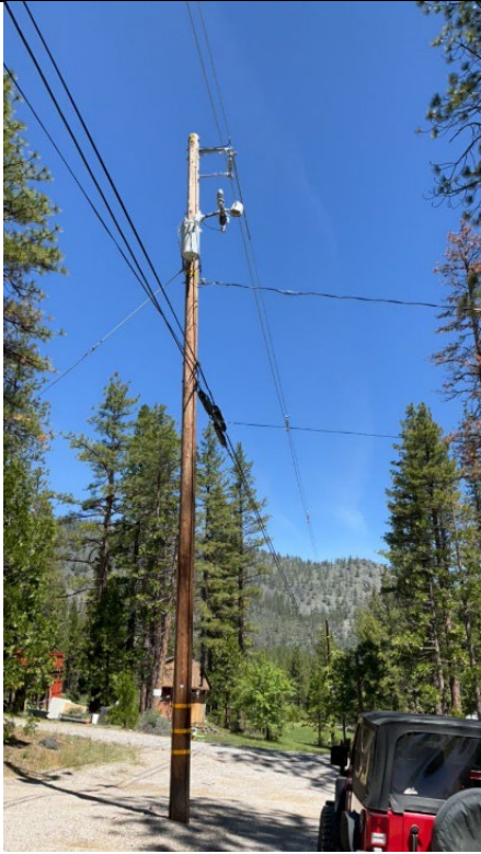
Item7IA1Img1: View of one line of covered conductor where two were reported.
