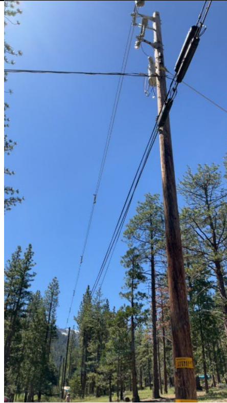
Item7IA1Img2: Another view of one line of covered conductor where two were reported.
